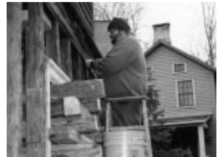
Volunteer Jeff Donat from Allentown Pa, removing siding from south wall of the mill.
