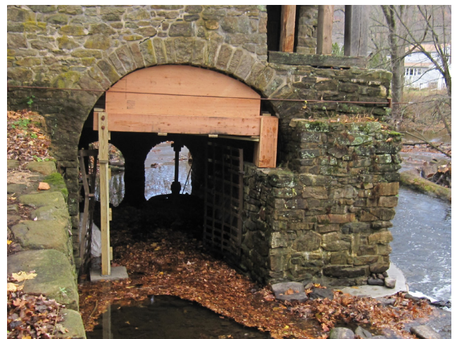
Emergency repair of the northeast corner foundation and intake arch that was completed September, 2016.
